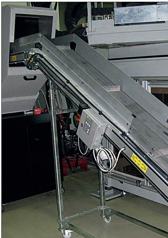
Installation example: Machinery protection. Plate type metal detector ELCON installed on the conveyor belt leading to the granulator. (old version)
